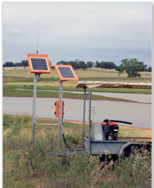
Remote pump management
