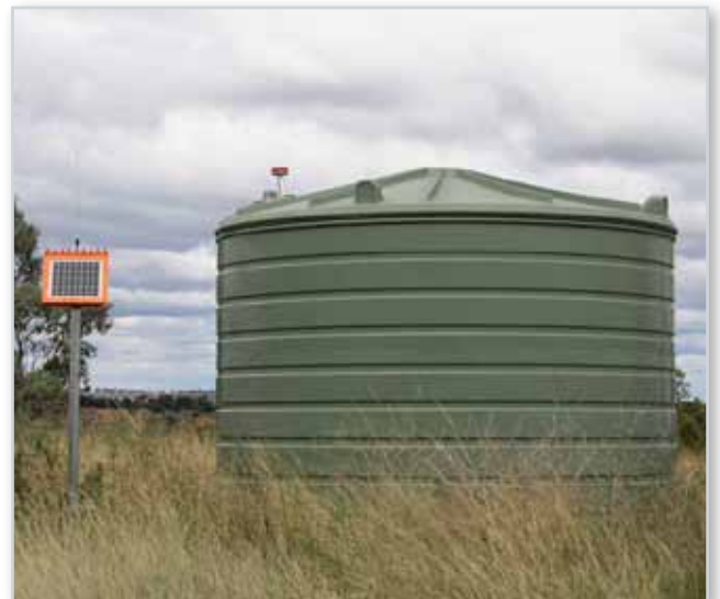
C2 water level monitoring solution Hartley Grazing Company, Mendooran NSW
