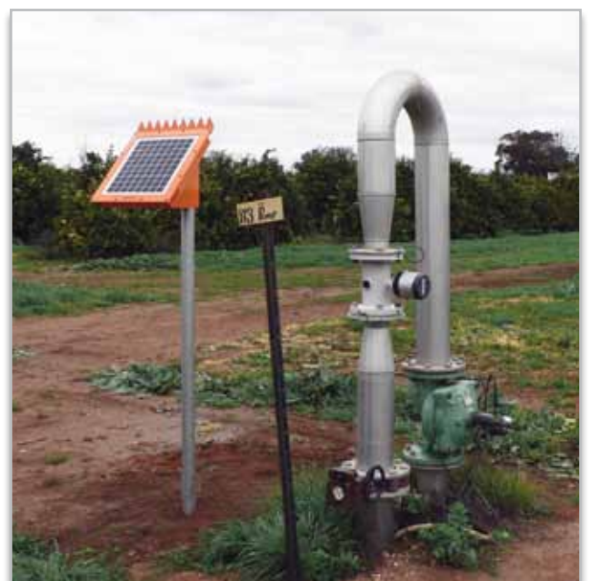
C2 water meter monitoring solution
